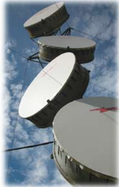
Telus Microwave Tower
