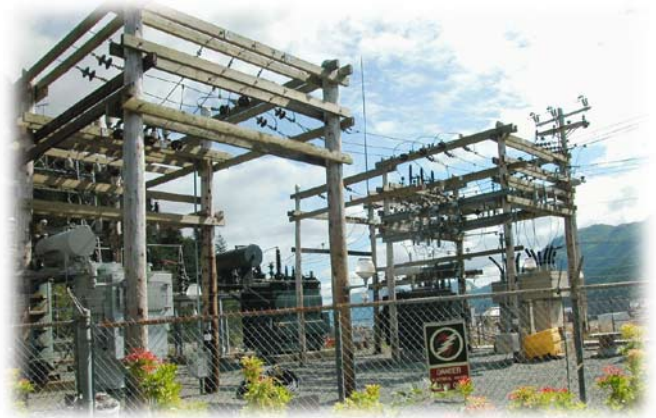
The BC Hydro Substation in Tahsis
